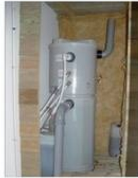
Figure 1. Basic greywater harvesting system. Water from baths, showers and laundry is to be reused for flushing WCs and watering the garden.
